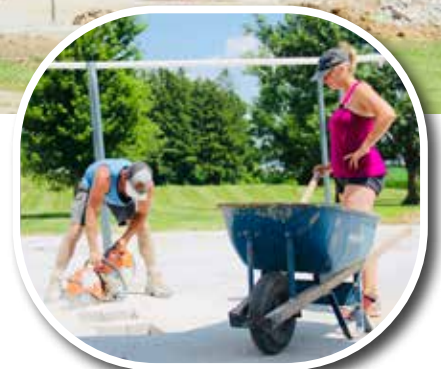
Blair Everman operates a concrete saw in preparation for placing a supporting pole for the new playground in Postville.
